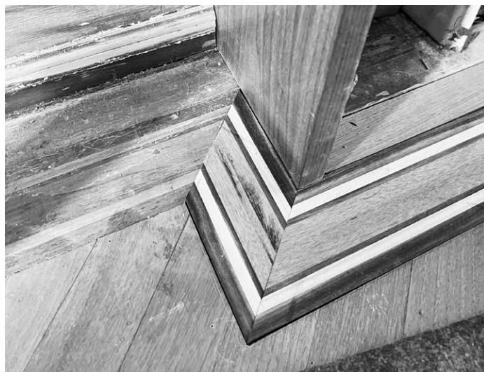
JB Book Mansion, Detroit, Michigan. Photo by John P. Biggar. Submitted by Integrity Building Group.
