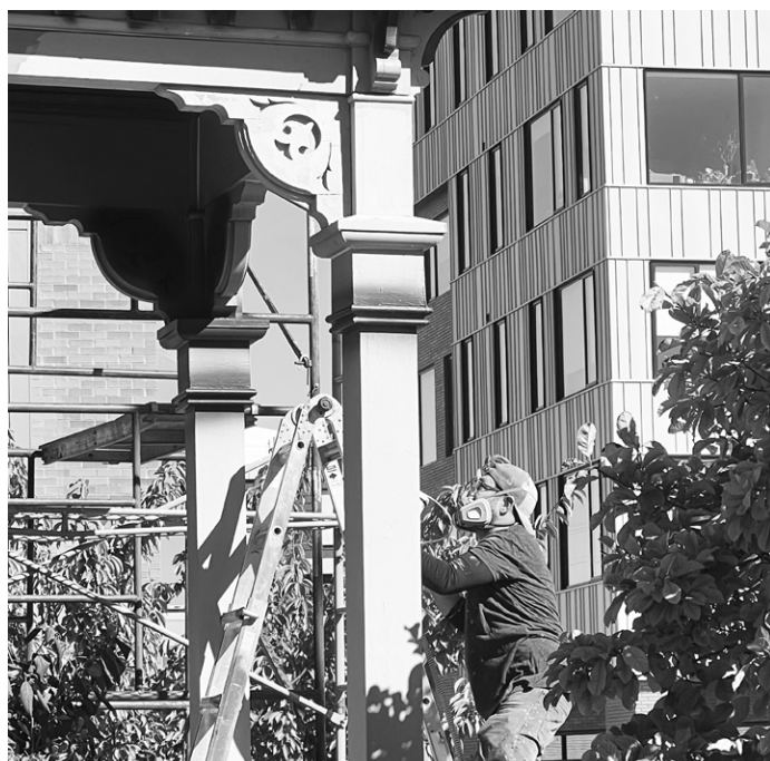
Brush Park Mansion, Detroit. Photo by John P. Biggar. Submitted by Integrity Building Group.
