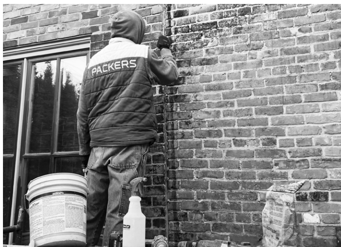
Brush Park Mansion, Detroit. Photo by John P. Biggar. Submitted by Integrity Building Group.
