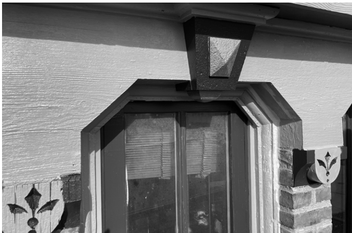
Brush Park Mansion, Detroit. Photo by John P. Biggar. Submitted by Integrity Building Group.
