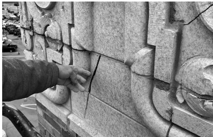
Music Hall, Detroit, Michigan. Photo by John P. Biggar. Submitted by Integrity Building Group.
