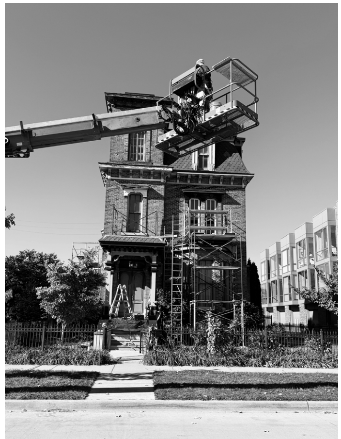
Brush Park Mansion, Detroit. Photo by John P. Biggar. Submitted by Integrity Building Group.
