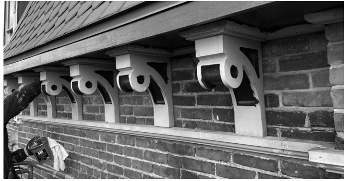
Brush Park Mansion, Detroit. Photo by John P. Biggar. Submitted by Integrity Building Group.
