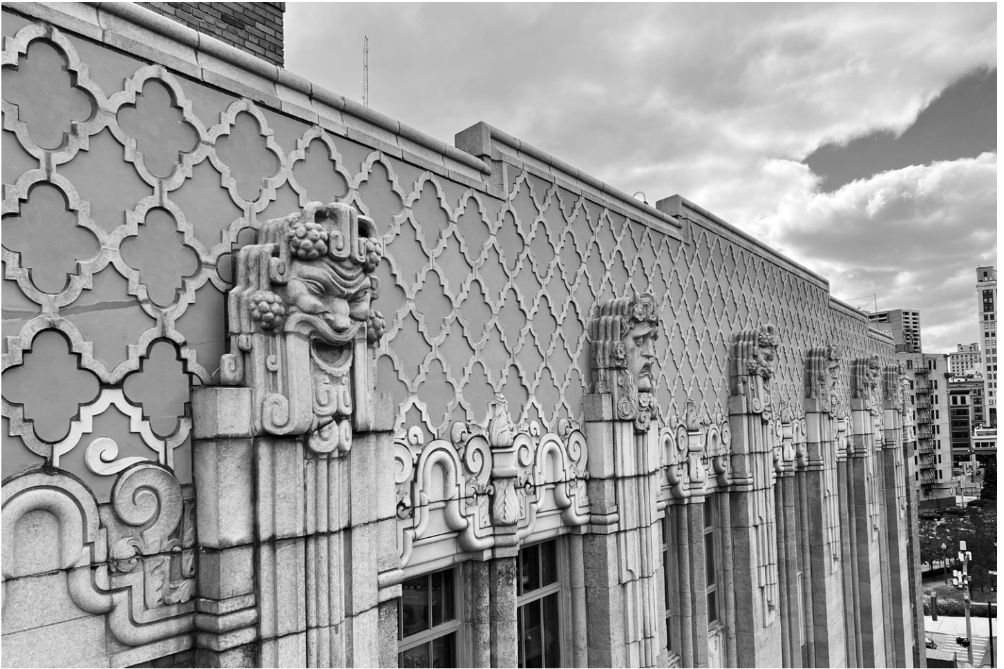
Music Hall, Detroit, Michigan. Photo by John P. Biggar. Submitted by Integrity Building Group.
