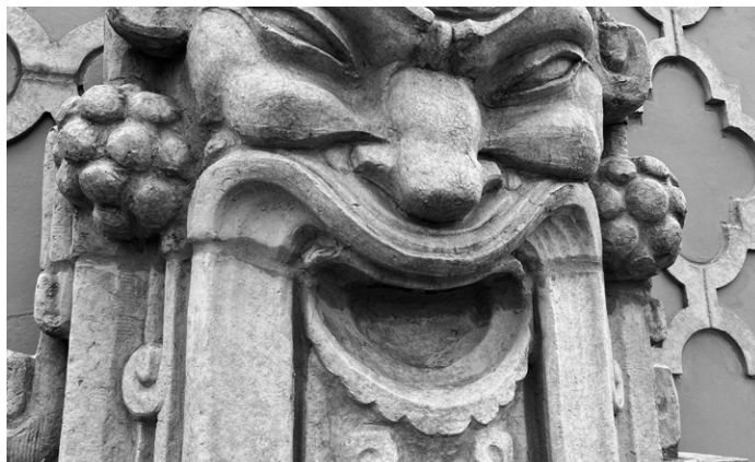
Music Hall, Detroit, Michigan. Restoration of the Corrado Parducci sculpture "masks". Photo by John P. Biggar. Submitted by Integrity Building Group.
