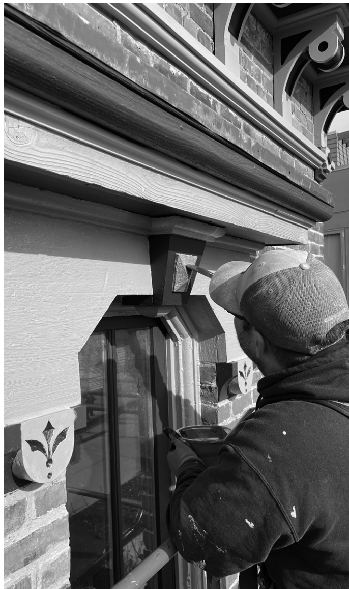
Brush Park Mansion, Detroit. Photo by John P. Biggar. Submitted by Integrity Building Group.
